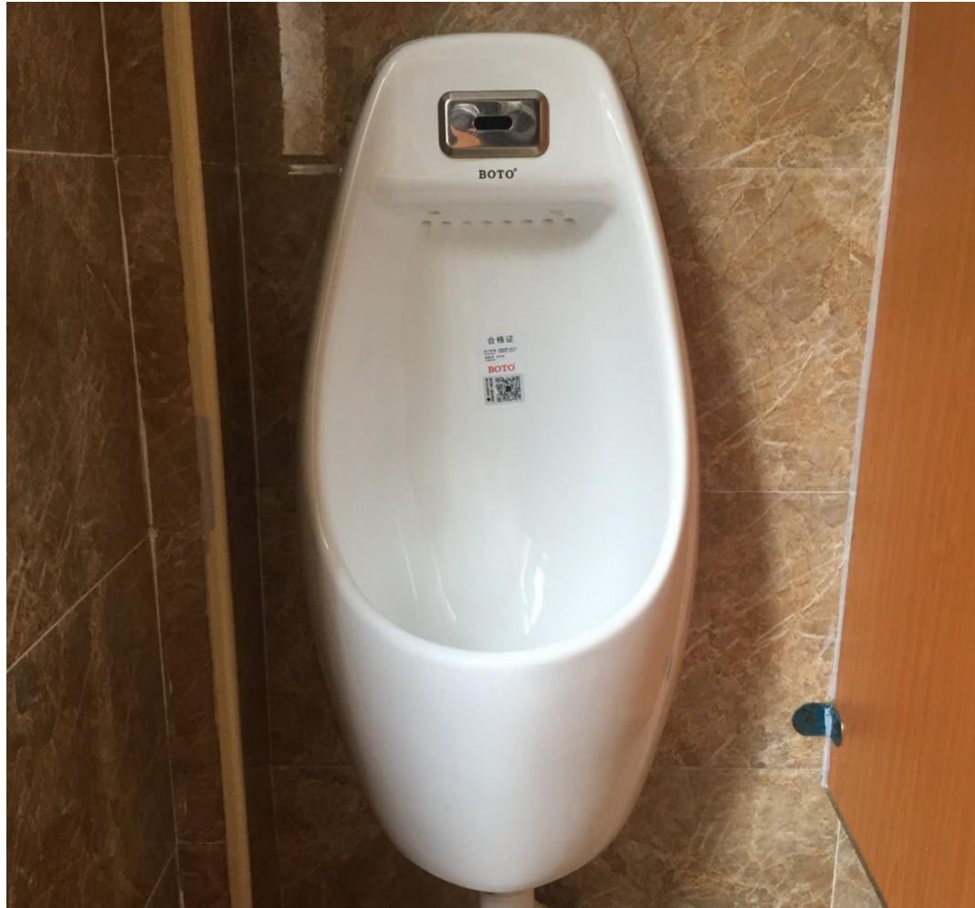
Photo of the urinal and its certificate of conformity
